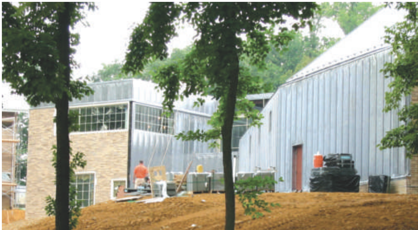
By late summer, construction work on the O'Brien Arts Center neared its final phase.
