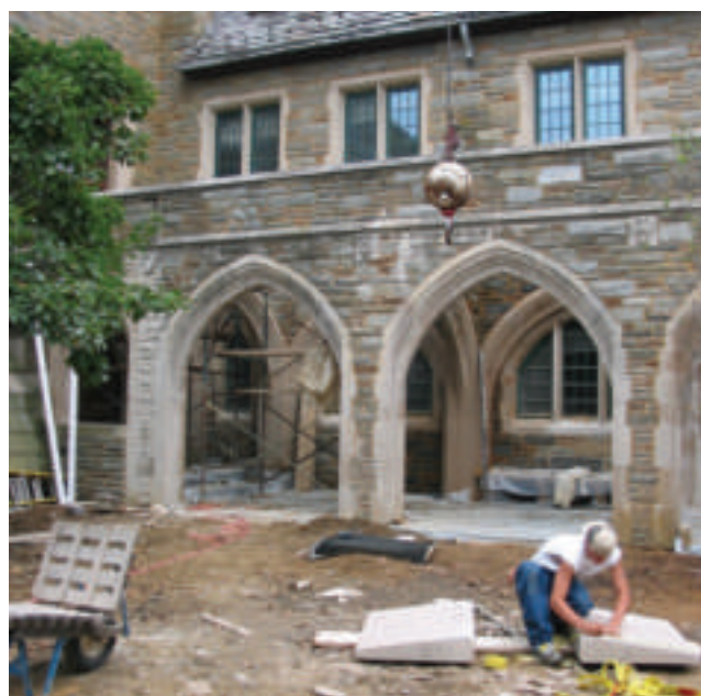
In addition to capping the stone arches of the Garth, the flagstones of the courtyard were refurbished and the underlying drainage structures were repaired.
