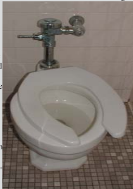
photo by Vivian Smith Moss toilets broken since 2003
